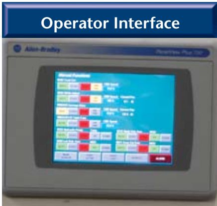
Operator interface (HMI) with color monitor. PLC sequence of operation.
